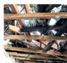
The damage left a gaping hole in their roof causing damage to belongings.
