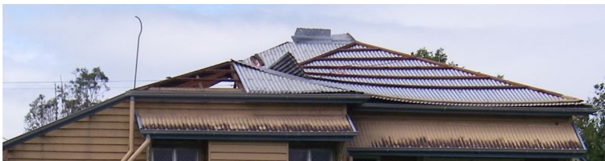
FIGURE 2. PART OF THE ROOF CLADDING WITH BATTENS STILL ATTACHED FLIPPED ON TO LEEWARD SIDE
