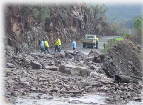
Events can be very destructive when roads or other infrastructure intersect with stormy weather in burnt and steep catchments. Some catchments represent higher risk than others. Photo: Adrian Murphy
